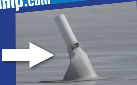
above: Vent damage from typical snow loads
